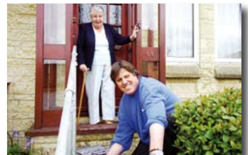
Chris Thorne from Care and Repair fitting a handrail for Mrs Fields from Bath, she says: "This hand rail will help me to be more independent."
